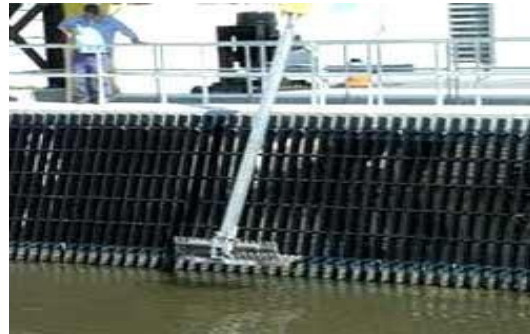
Trash rack for collecting trash and debris
